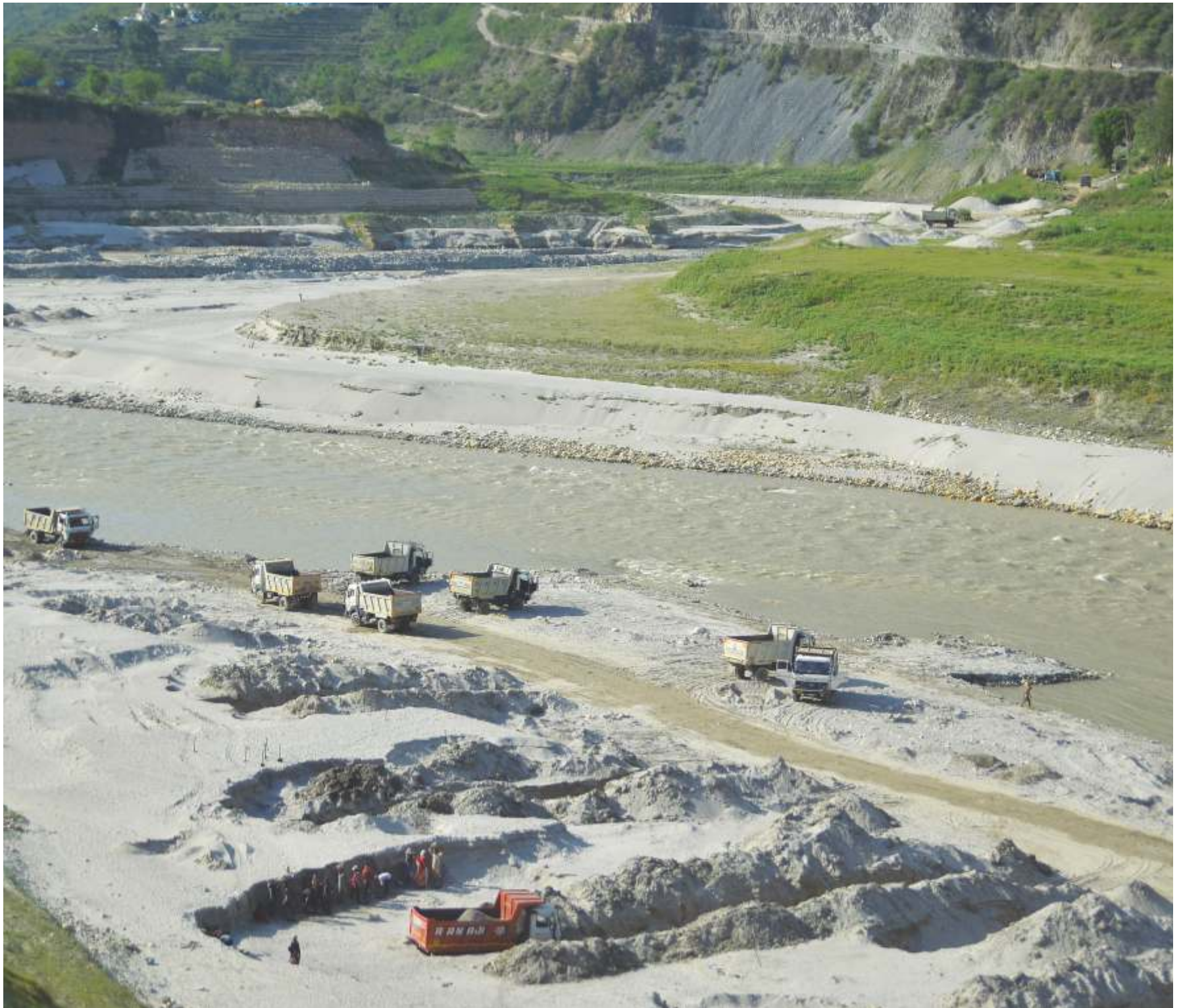
Unveiling Earth's Treasures: Explore the sand mining in Ganga, where nature's geological riches are responsibly harnessed to shape construction and growth, Gangotri, Uttarakhand.
